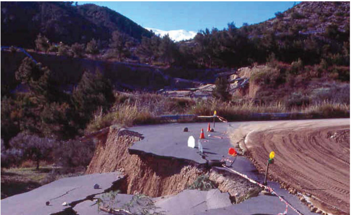
Figure 4 (c) – Infrastructure and building problems in broader Rio area due to landslides, coastal erosion and poor development design.
