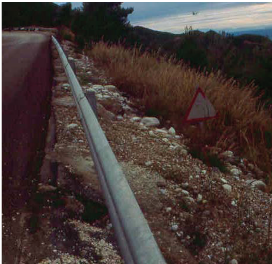
Figure 5(b) – Old sign next to a road built on an active landslide. The road was repaved, but the sign indicates that the landslide is still active.
