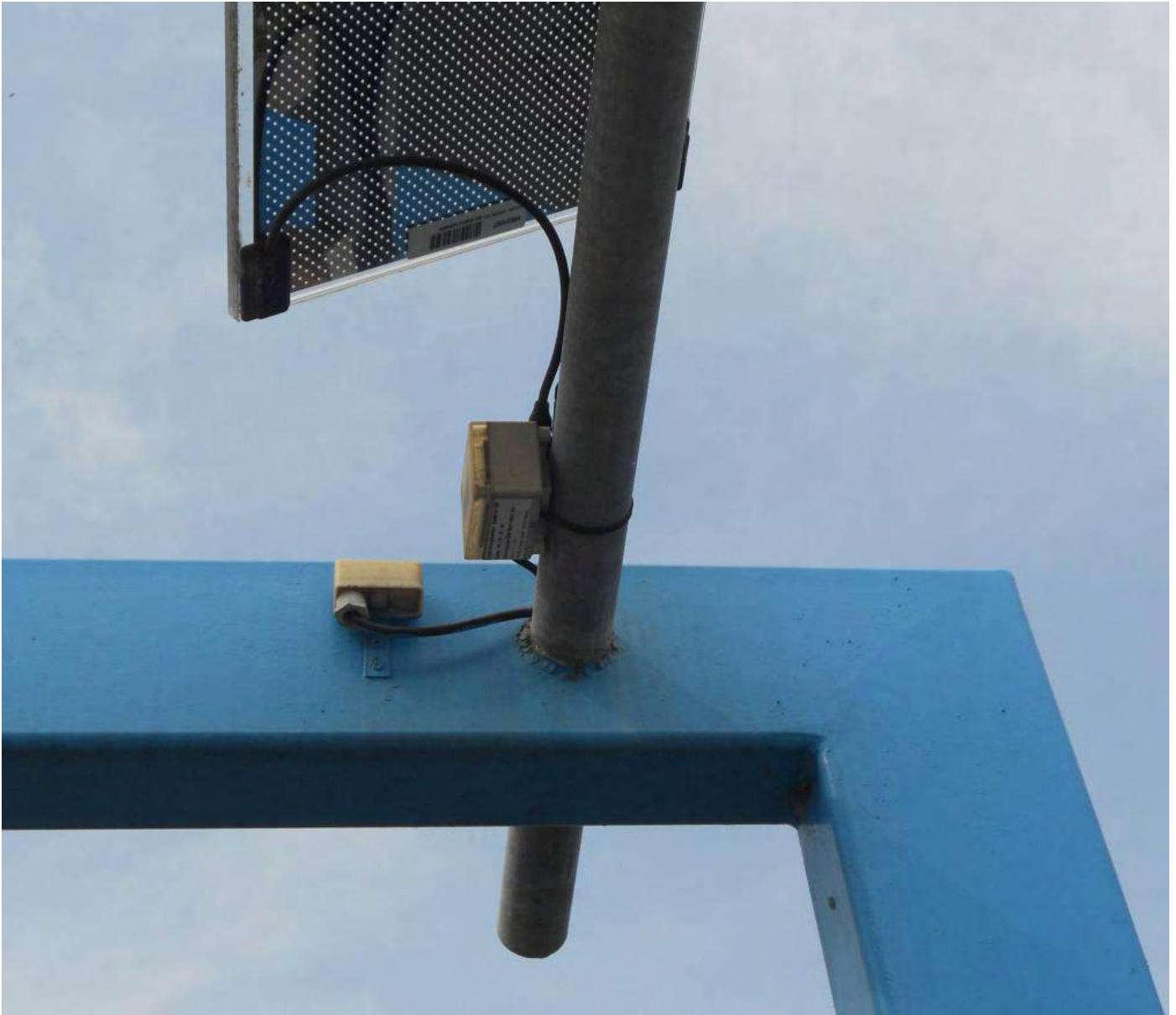
Figure 3 – Ameglia (La Spezia, Italy). Detail of photovoltaic trellis wiring. Five 2.40 m x 0.30 m module strips for each pergola facing south / east at an angle of 30 ° above the horizon, support the semi-transparent thin film with a pattern of 10% of holes which produce up to 240 Wp (photo R. Valente).
