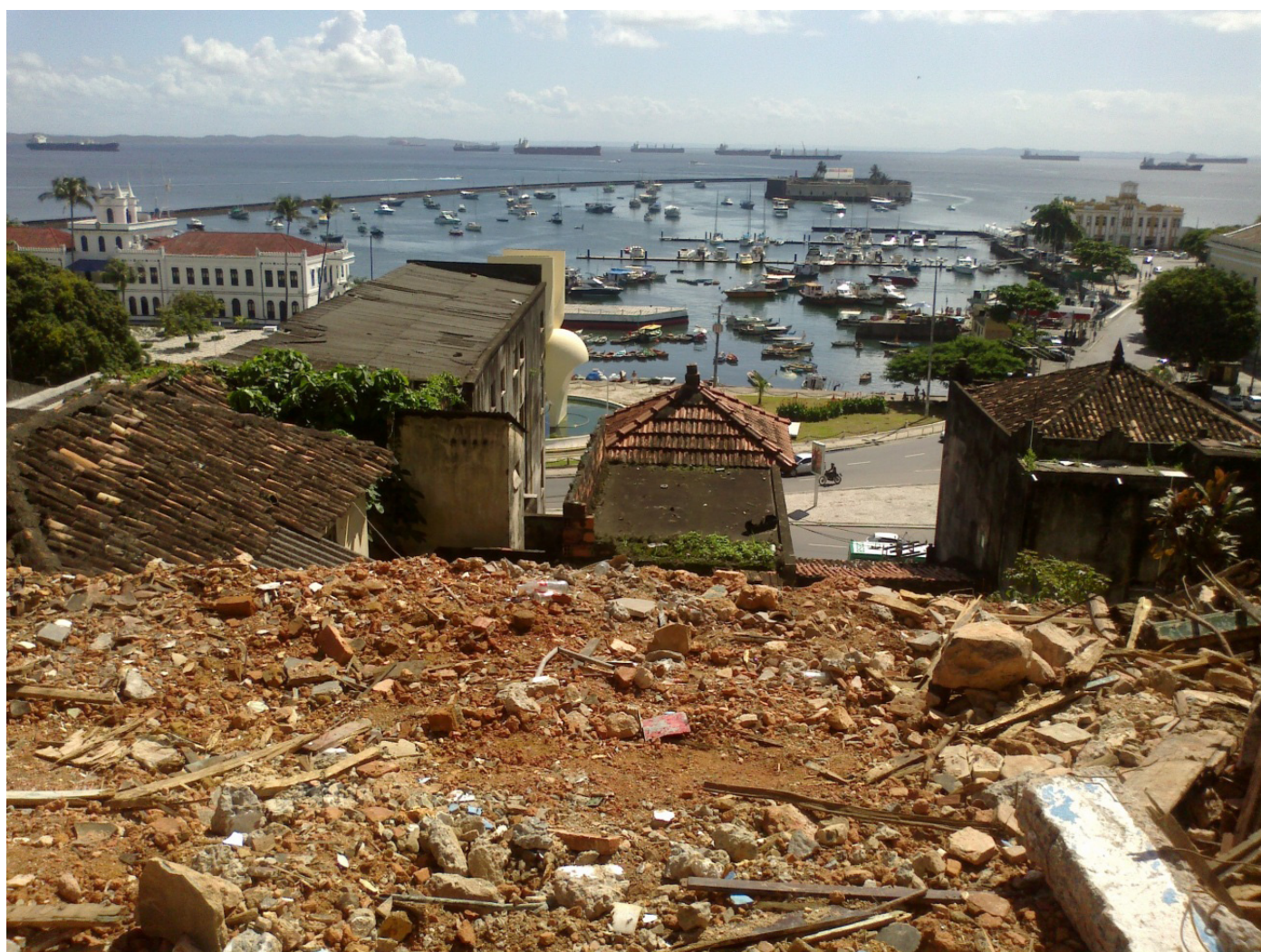
Figure 9 – Historic Center of Salvador: demolitions of sets of properties in Ladeira da Montanha, carried out in May 2015 by the Civil Defence Body of Salvador City Hall (CAU-BA Archives, 2015).
