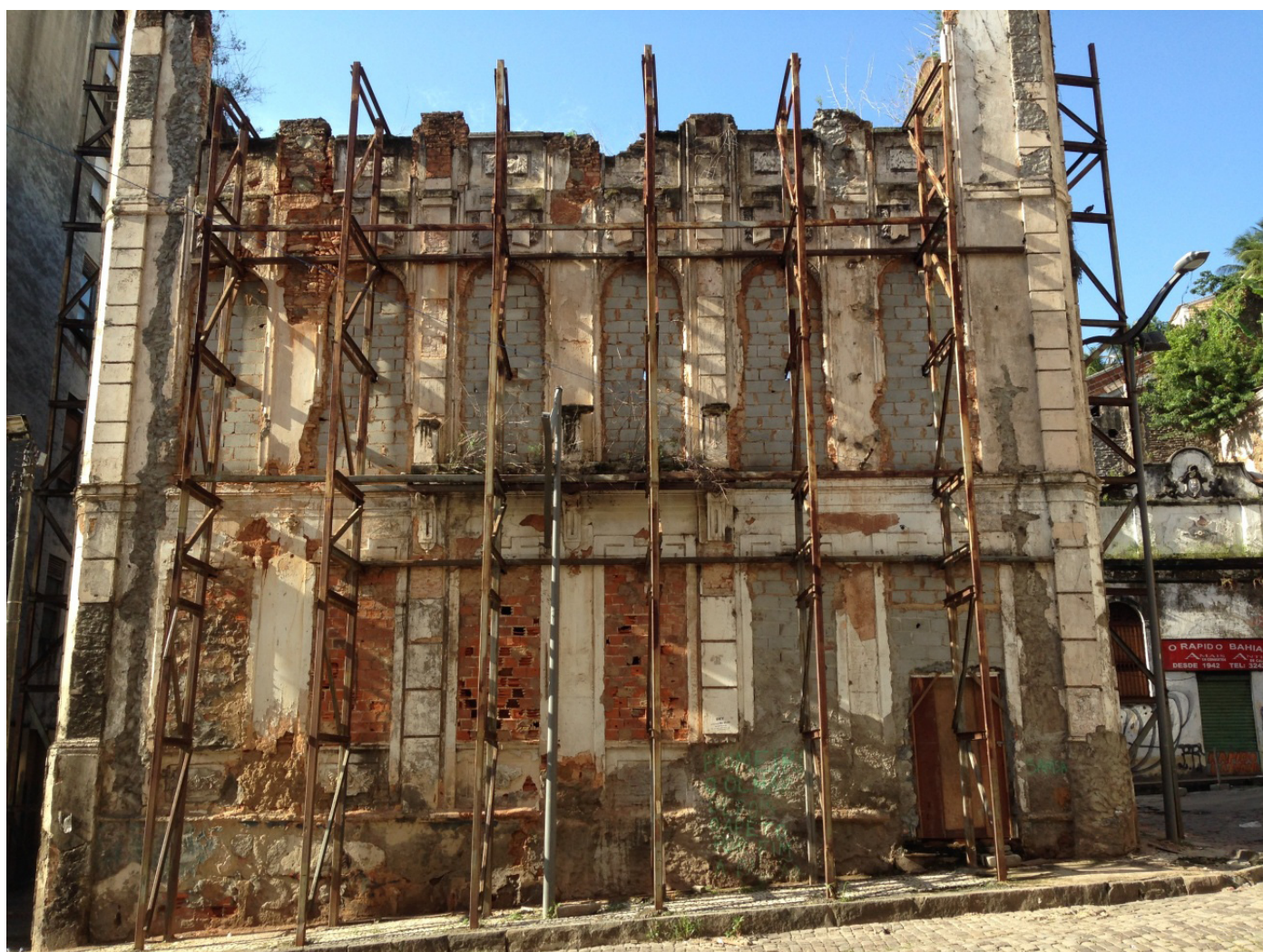
Figure 7 - Historic Center of Salvador: shored-up ruin in Taboão Street (Nivaldo Andrade, 2015).
