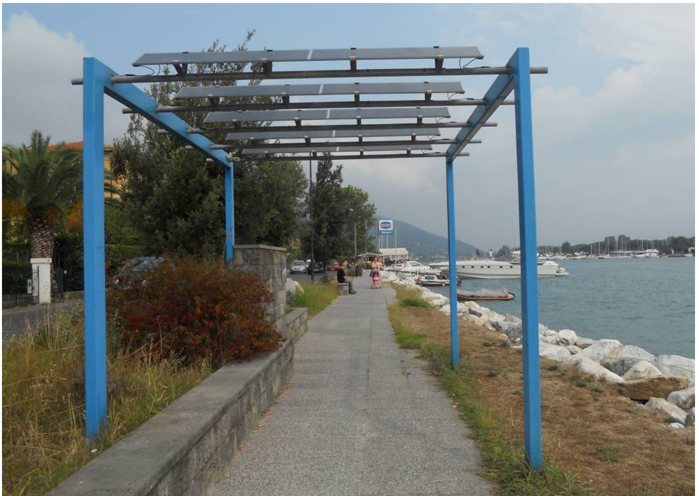
Figure 2 - Ameglia (La Spezia, Italy). One of three prototypes of stand-alone photovoltaic shelter made in 2004, as part of the Italian German PVACCEPT research project funded by the European Commission. This project is based on the integration in the architectural historic environment and landscape (photo R. Valente).
