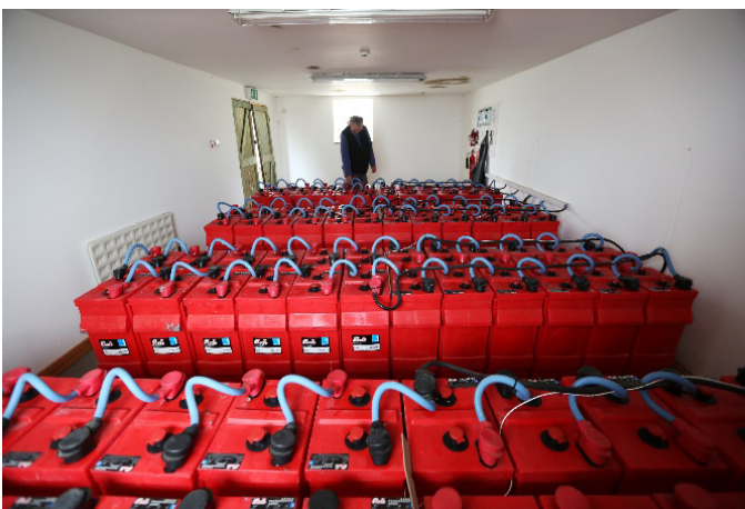
Eigg Electric, Centre for energy storage, Isle of Eigg, Scotland, 2008.
