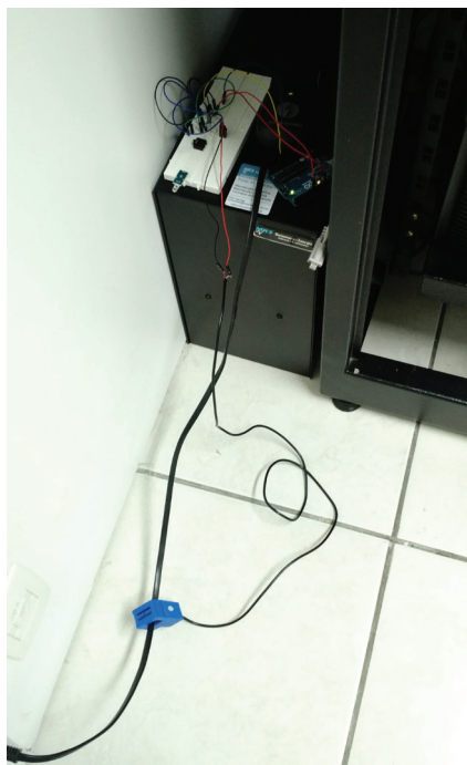
Figure 6 – Developed system collecting data from the Data Center.
