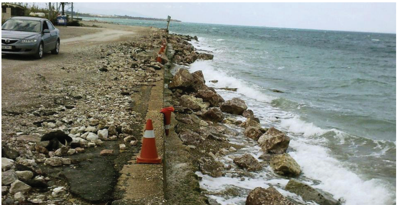
Figures 3 (a) and (b) – Partial view of a coastal road in Rio city. The signs of erosion and coastal retreat are evident.
