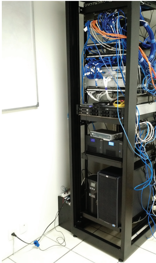
Figure 5 – Non-invasive current sensor (100A SCT-013) collecting data from the Data Center.
