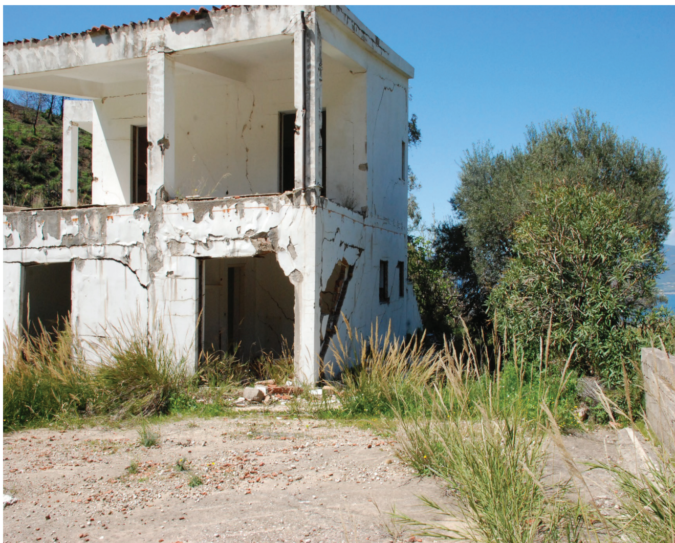
Figure 4 (a) – Infrastructure and building problems in broader Rio area due to landslides, coastal erosion and poor development design.
